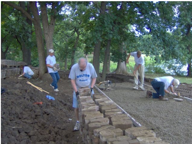
Floyd Gruver (center) and Tom Routh (2 nd from l.) carry patio blocks at a work day at Lake Shawnee while county employees prepare a patio area at the right.
